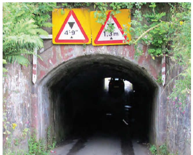
This tunnel near Kirkintilloch, Scotland could well be Britain’s smallest road tunnel
